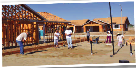
Participant families hard at work on their new homes in Goshen. Top Right: Families receive certificates of completion.
