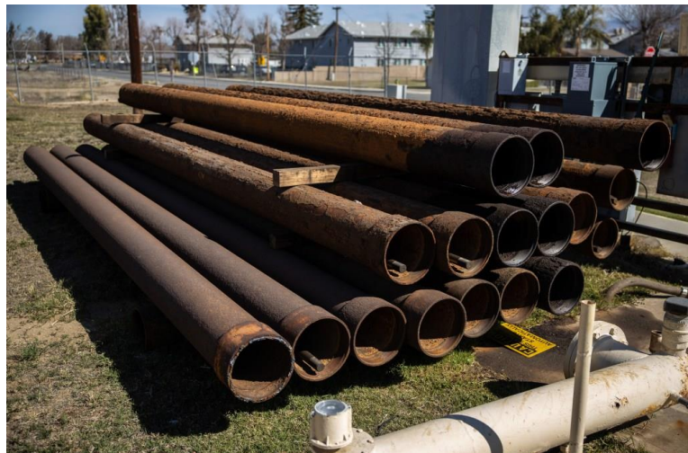
Defunct well water pipes stacked at the Lamont Public Utility District Well #13, which recently broke because of age. The district is waiting on funding to fix several of its wells so it can consolidate with nearby El Adobe.
