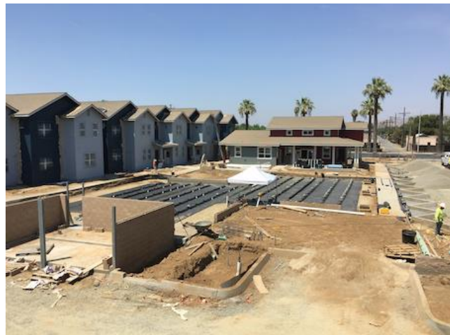
At an installation site in California, storm water from adjacent areas is captured, stored and reused for irrigation.
