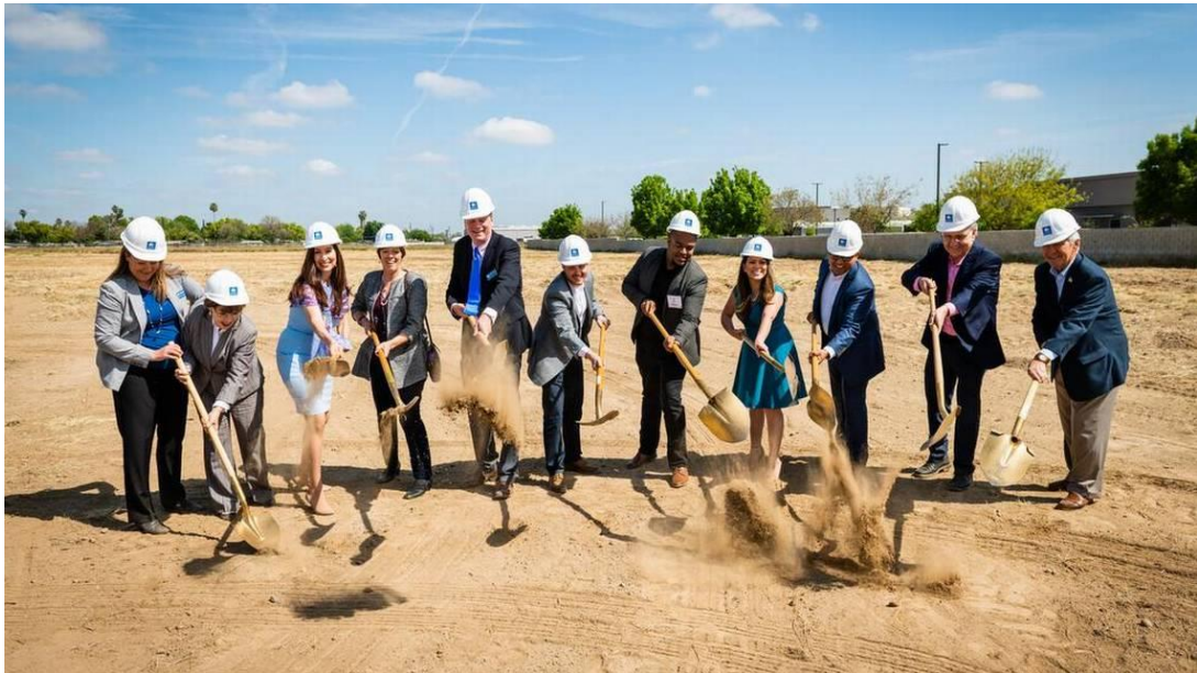
Congressman Costa, City of Fresno Mayor Brand, Council VP Arias and Councilmember Soria, along with many representatives from Wells Fargo, Clinica Sierra Vista and more during the groundbreaking ceremony of Annadale Commons, a senior affordable rental community in South West Fresno on April 12.
