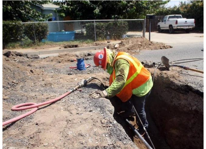
A construction worker uses a machine to burrow piping for water connectivity to a house on Page Street in east Porterville on August 23, 2017. Hundreds of households are receiving free connectivity through state, federal and local funding. Daniel Casares- dcasarez@vidaenelvalle.com
