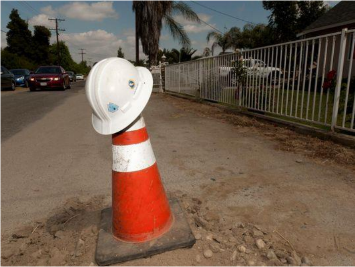
Cal Water and the local rotary clubs hold a ground breaking Thursday, April 28, 2016 on Avenue 322 east of Highway 63 for a water project that will bring water to 14 county residents in the area whose wells have run dry. Some have been without water for nearly two years.
