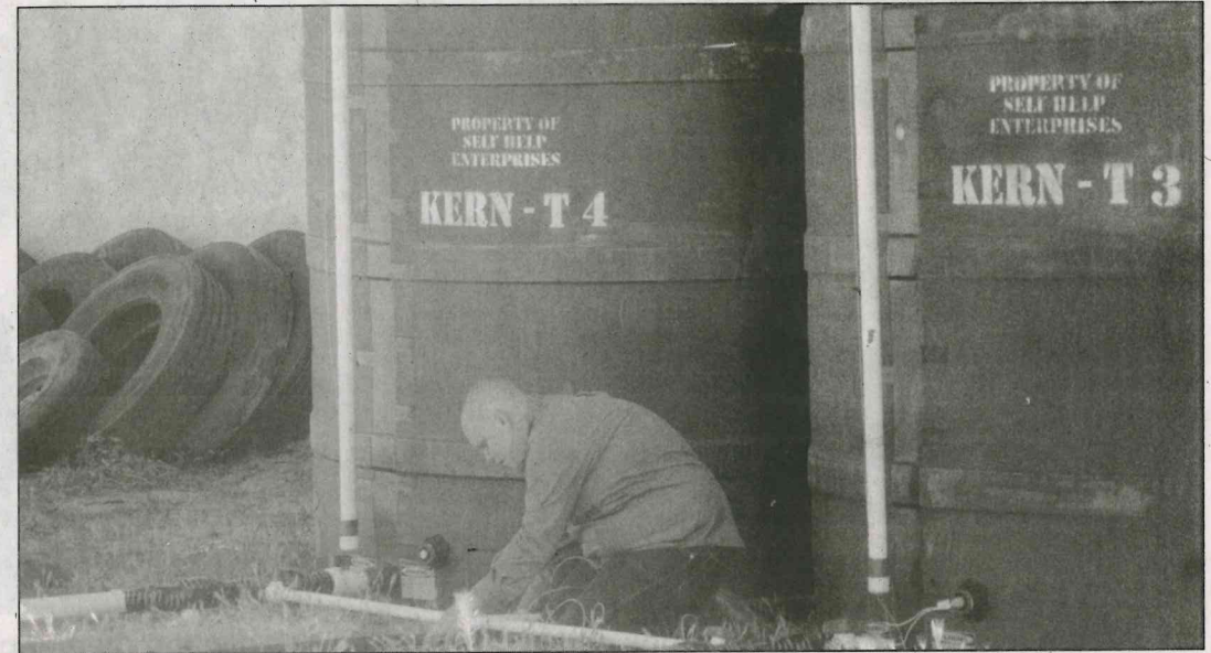
The two tanks will be hooked up to a pump that will get the water into the houses.
