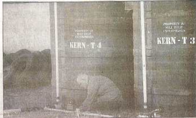
The two tanks will be hooked up to a pump that will get the water into the houses.
