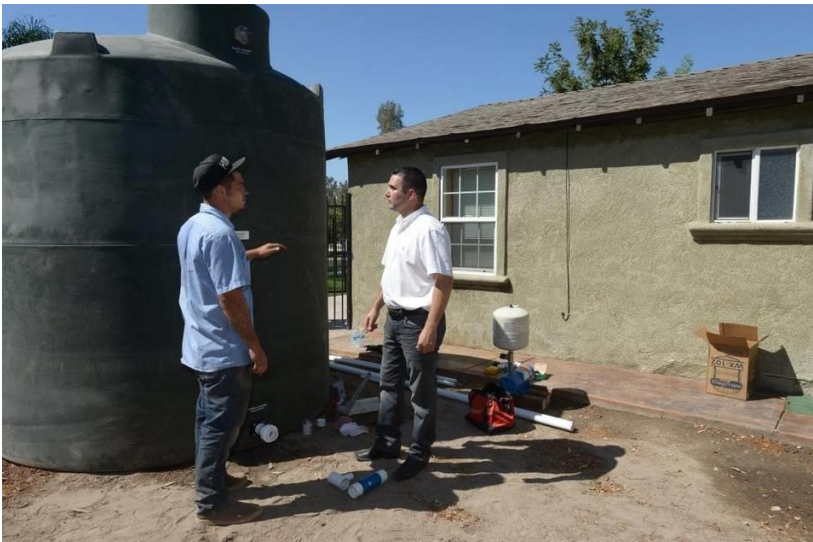
Homeowner Genaro Gil, right, speaks with installer Bryce Bryant on Tuesday in Ceres about the temporary water storage system he will have until he gets a new well. An installation team with Wilkins Pump brought and installed the large tank that will stay next to the house.
