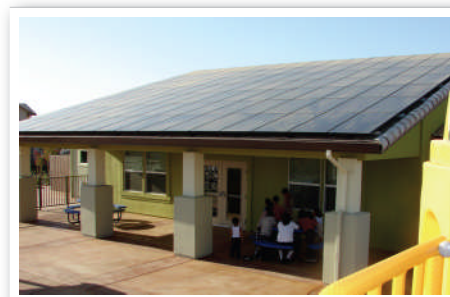
A 42,000 kWh solar system provides the energy needs for the community center and communal lighting
